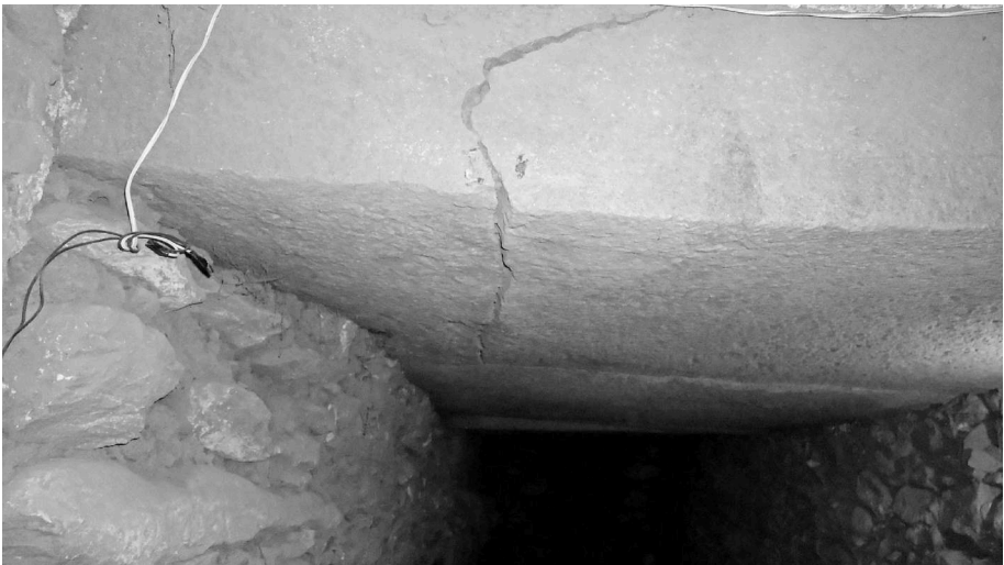
Fig.5: Crack on a roof lintel of the mausoleum as observed in 2012 (Photo by Tekle Hagos)
