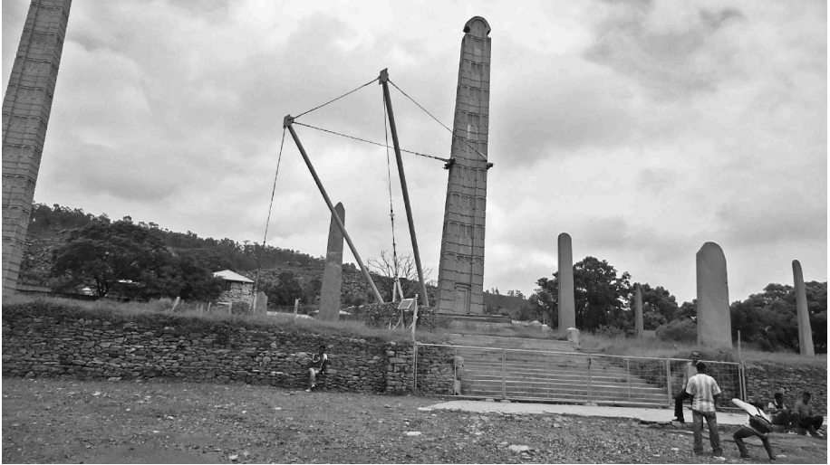
Fig.2: Stela 3 tied with cables during 2008 during reinstallation process. (Photo by Tekle Hagos)
